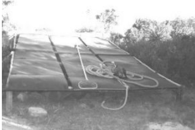
Figure 2: Pool solar water-heater
