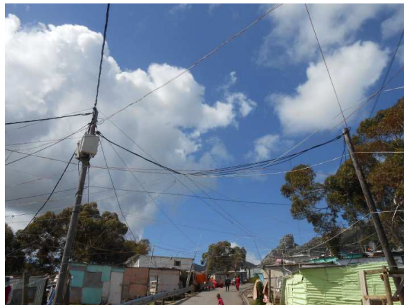
Figure1: Formal and informal electricity lines in Imizamo Yethu. The black lines are formal and are connected to the municipal distribution box
