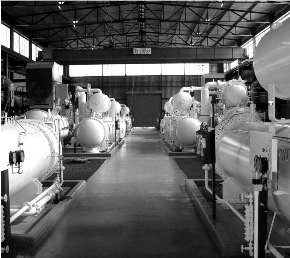
Figure 1: Chiller room at a large industrial plant
